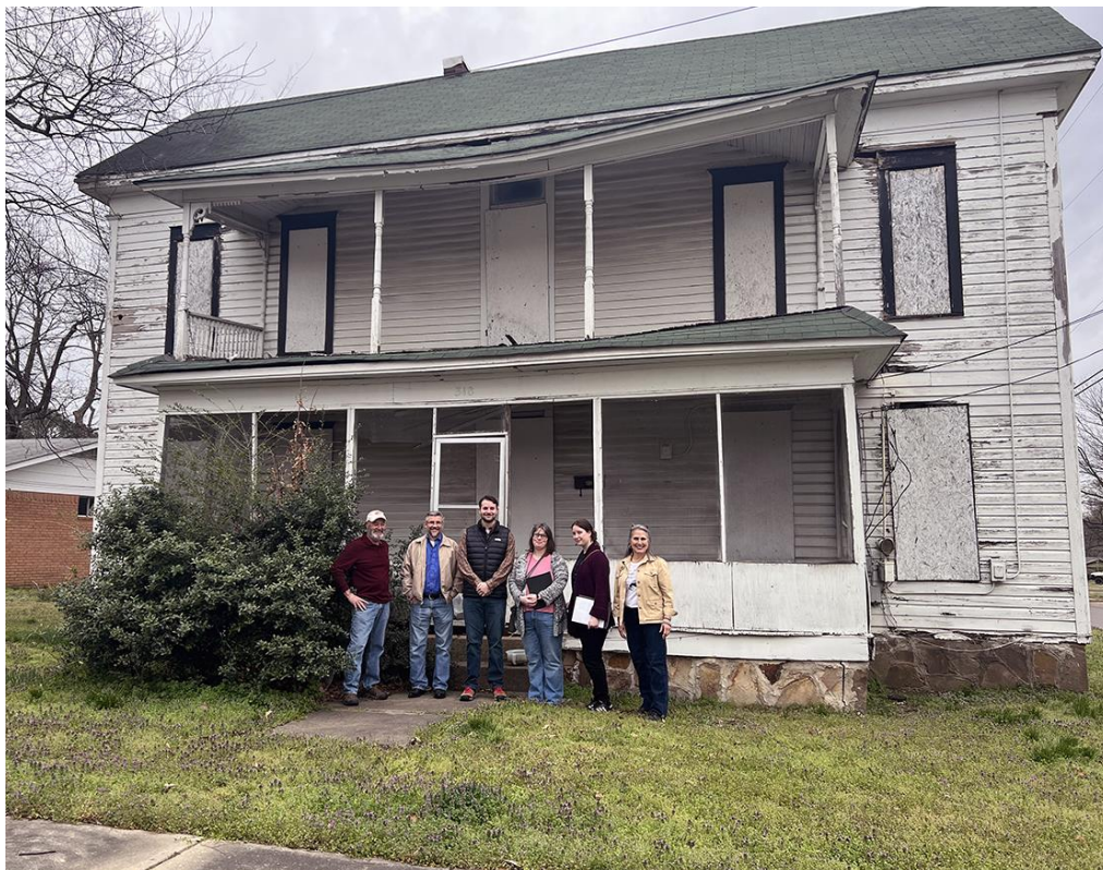
AHPP Technical Services and Federal Programs Staff on a site visit to the Latimore Tourist home in Russellville, Ark.
