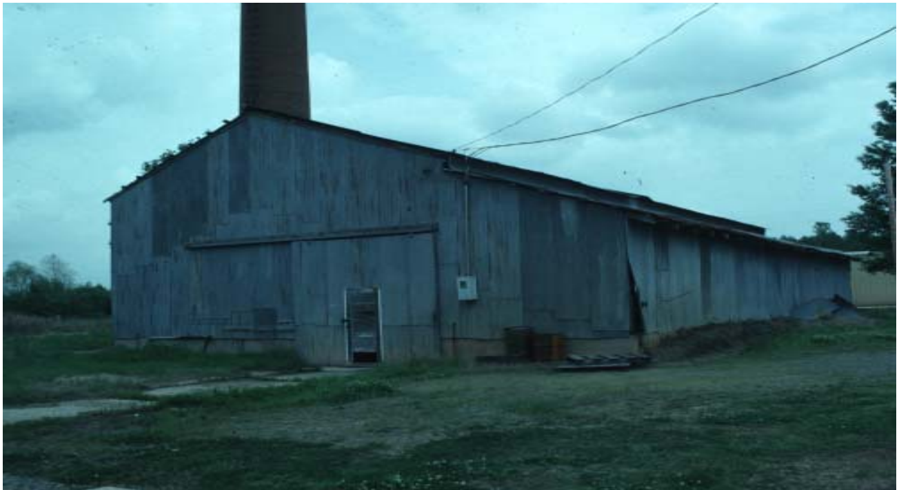
The boiler house and its looming brick smokestack still survive at the Rohwer Relocation Center site. (Arkansas Historic Preservation Program file photo)
